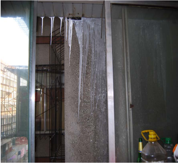
Icicles like this are very dangerous and likely to harm residents
